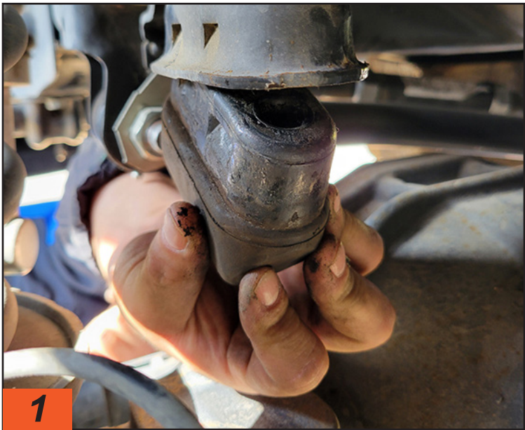
The first step for installing the front springs was to remove the original bump stop from the frame on both sides the truck. A screwdriver was used to release the edge of the bump stop, which then came out by hand.
