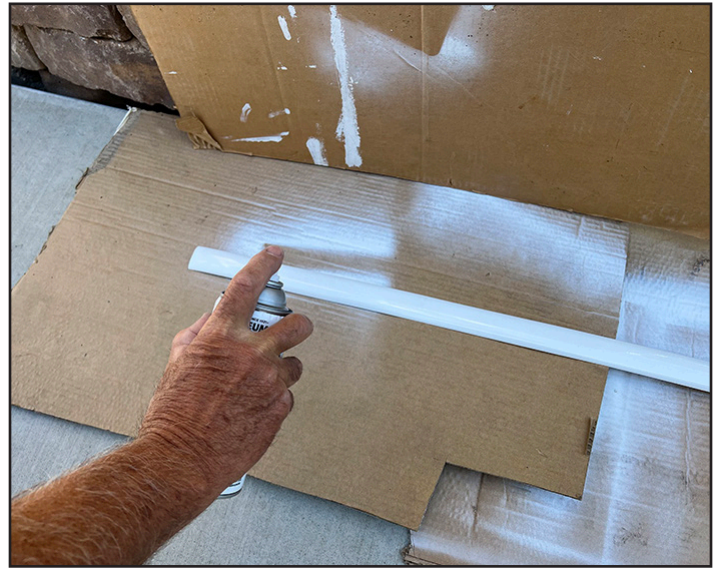
White spray paint was used to restore the molding color. Always spray light coats to prevent the paint from running. The paint was allowed to dry overnight.
