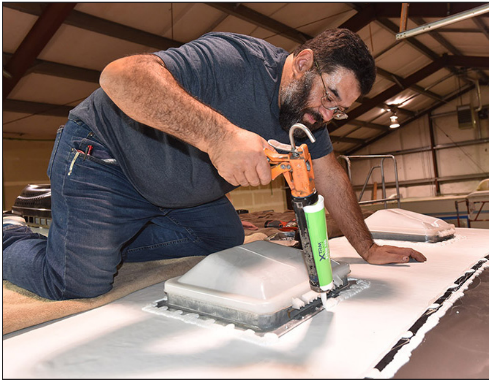
Carrier RV's Tony Salazar re-seals vents and roof cap molding on a customer's trailer using self-leveling sealant.
