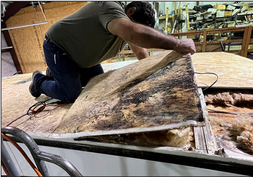
The rear corner of this trailer's roof decking was rotted from a leak in the TPO that wasn't discovered until the owner saw a blister on an interior ceiling panel many months after the damage had occurred.
