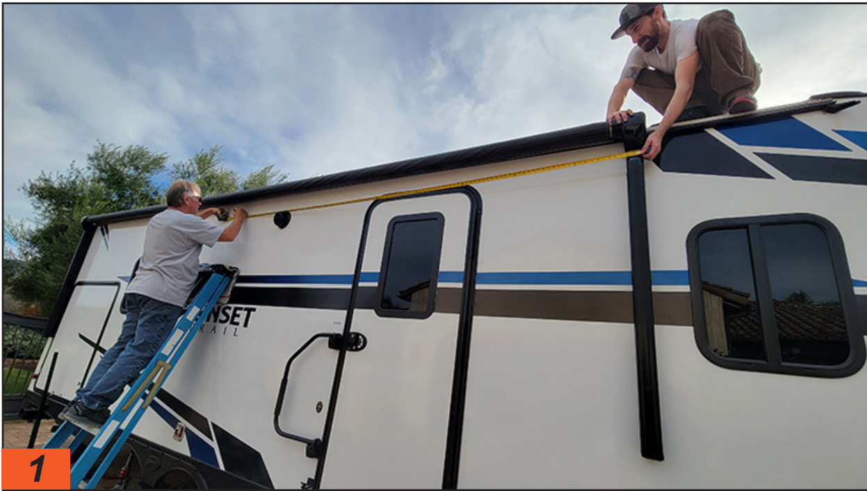
1 The first step is to locate the center of the awning tube. Here the awning spans almost the entire length of the trailer, making the cradle assembly necessary to prevent sagging.
