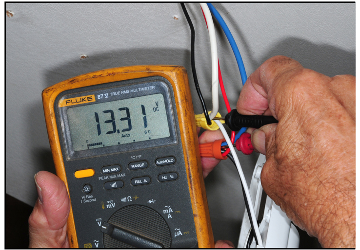
Direct current (12-volt DC) powers most of the lights, the furnace, demand pump and refrigerator control module, to name a few items. The light fixture here was erratic so the power was checked with a multimeter. There was plenty of power to the fixture, so the light failed.
