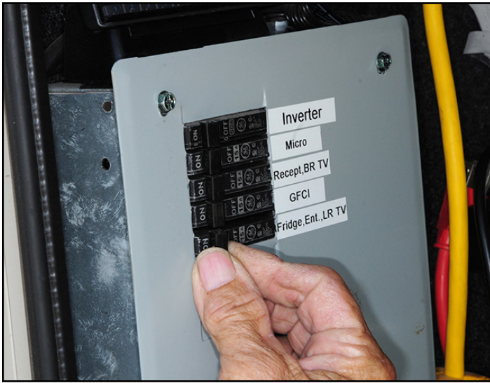
RVs equipped with larger inverters (usually 2,000 watts and higher) will have subpanel with additional breakers mounted near the main distribution panel. Sometimes owners forget about this panel and are dumfounded when diagnosing an electrical outage.
