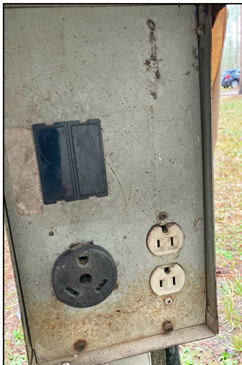
Many campground owners perform little or no maintenance on their pedestals, resulting in poor electrical connections that can melt the shore power cord or create a hot-skin condition. Note that this one has eliminated the circuit breakers, a clear violation of the National Electrical Code (NEC).
