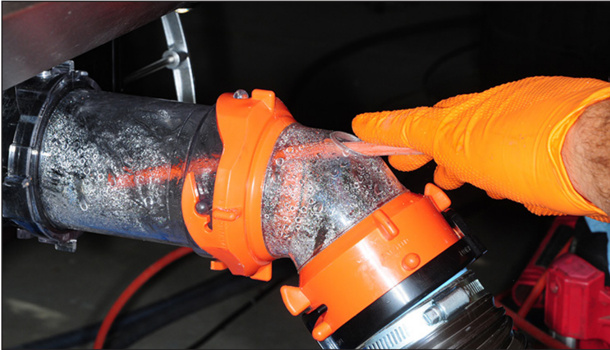
Pressure-cleaning holding tanks should be part of your annual RV maintenance.
