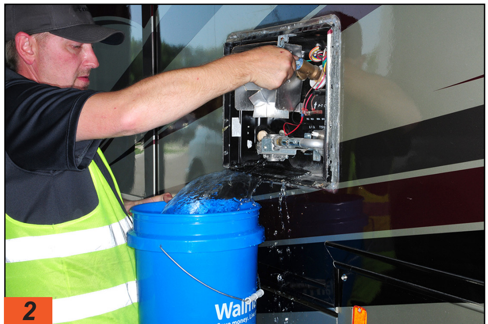
2 Once the original water heater was turned off and allowed to cool down, the drain plug was removed and the pressure-relief valve opened to empty the water from the tank into a bucket.
