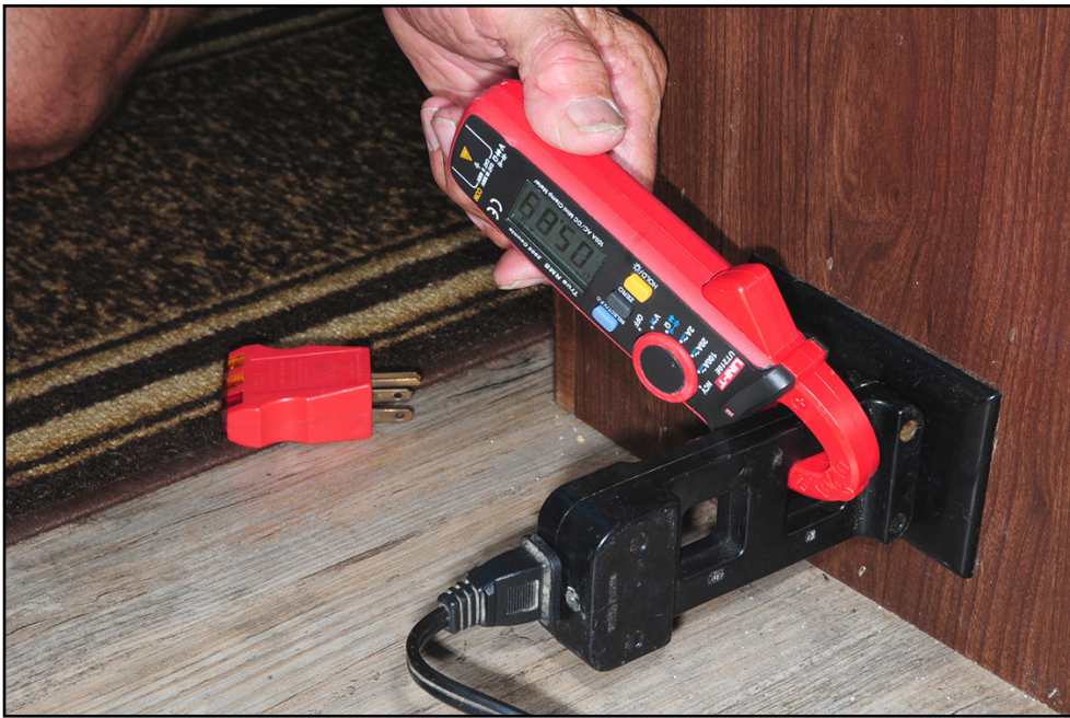
An amp meter (shown here) or multimeter with a clamp-on induction ring makes it easy to test for low or high amp draw. An adapter can be used in lieu of spreading the wires for testing. The induction clamp can only read one wire.
