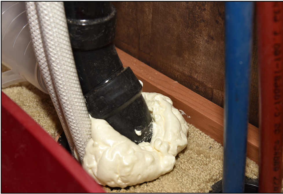
Here is a good example of how to properly seal a sink drain. First the area around the pipe was stuffed with steel wool, then spray foam was sprayed on top and around that. This is to prevent rats and mice from chewing through the foam and crawling in the bathroom from underneath your RV.
