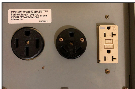
A modern Class-A GFCI outlet is designed to trip with a fault current over 5 mA. It's a good test of normal leakage currents in your RV's electrical system.
