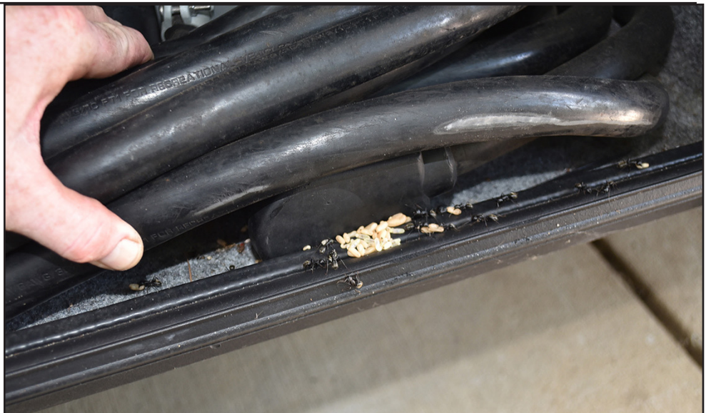
Nothing will spoil a trip faster than discovering your electrical bay has turned into a playground for hundreds of carpenter ants. Notice the white eggs that are everywhere. Luckily this infestation was caught before major damage was done.
