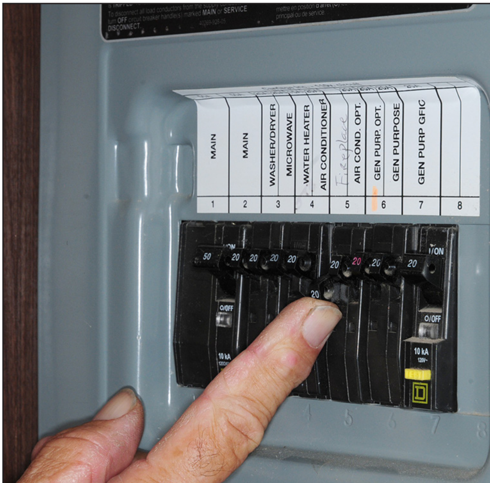
You can identify the 120-volt AC distribution panel by the home-style circuit breakers that snap into a frame. There are a few different styles that are used for this purpose. Circuit breakers wear over time, depending on how often they are tripped. Replacements are easily found in hardware or home supply stores.
