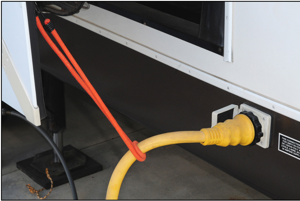
Power cords that are connected to the side of the RV need some type of strain relief to prevent premature failure. Here, a bungee cord is attached to the slide-out frame and does a good job of reducing strain.
