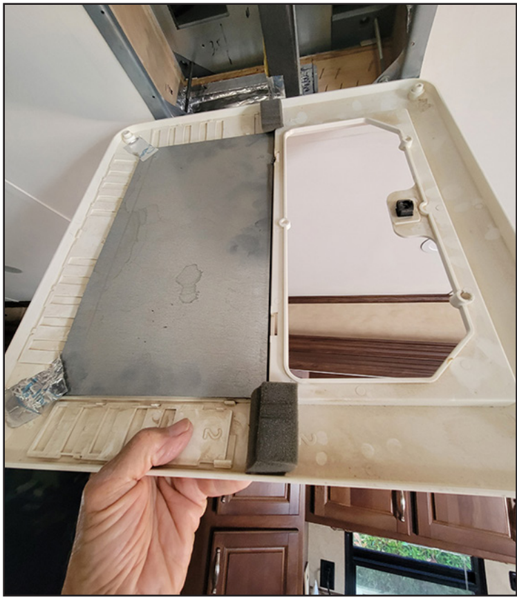
Once the ceiling assembly was removed it was immediately clear that the airflow was restricted because of the way the plenum was designed and the configuration set by the factory.
