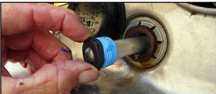
Wrap the anode rod threads with Teflon tape before reinstalling it into the tank. Tighten with a good amount of torque.
