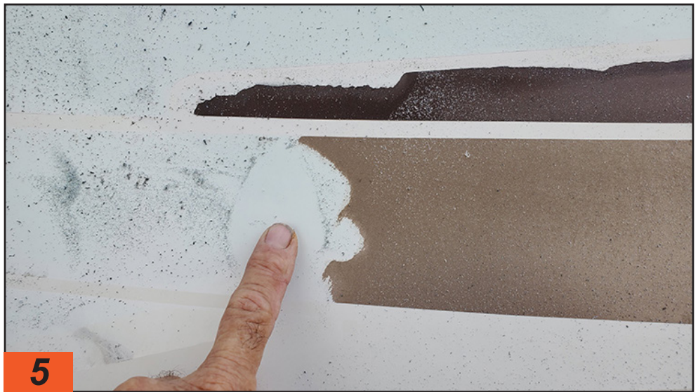
The removal wheel makes short work of grinding the vinyl from the sidewall, without damaging the surface. Still, the entire job takes a lot of patience.
