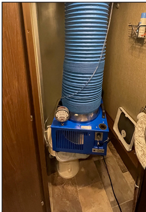
The Sealtech unit is usually set up under a 14 x 14-inch roof vent. It brings in outside air to pressurize the RV body.
