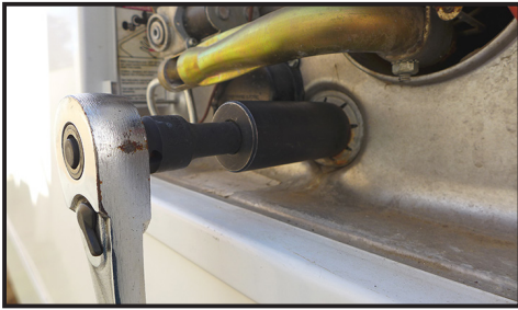
Removing the drain plug/anode rod in a water heater requires the use of a 11/16-inch deep socket, short extension and ratchet. You may need a breaker bar if the plug/rod is tight.
