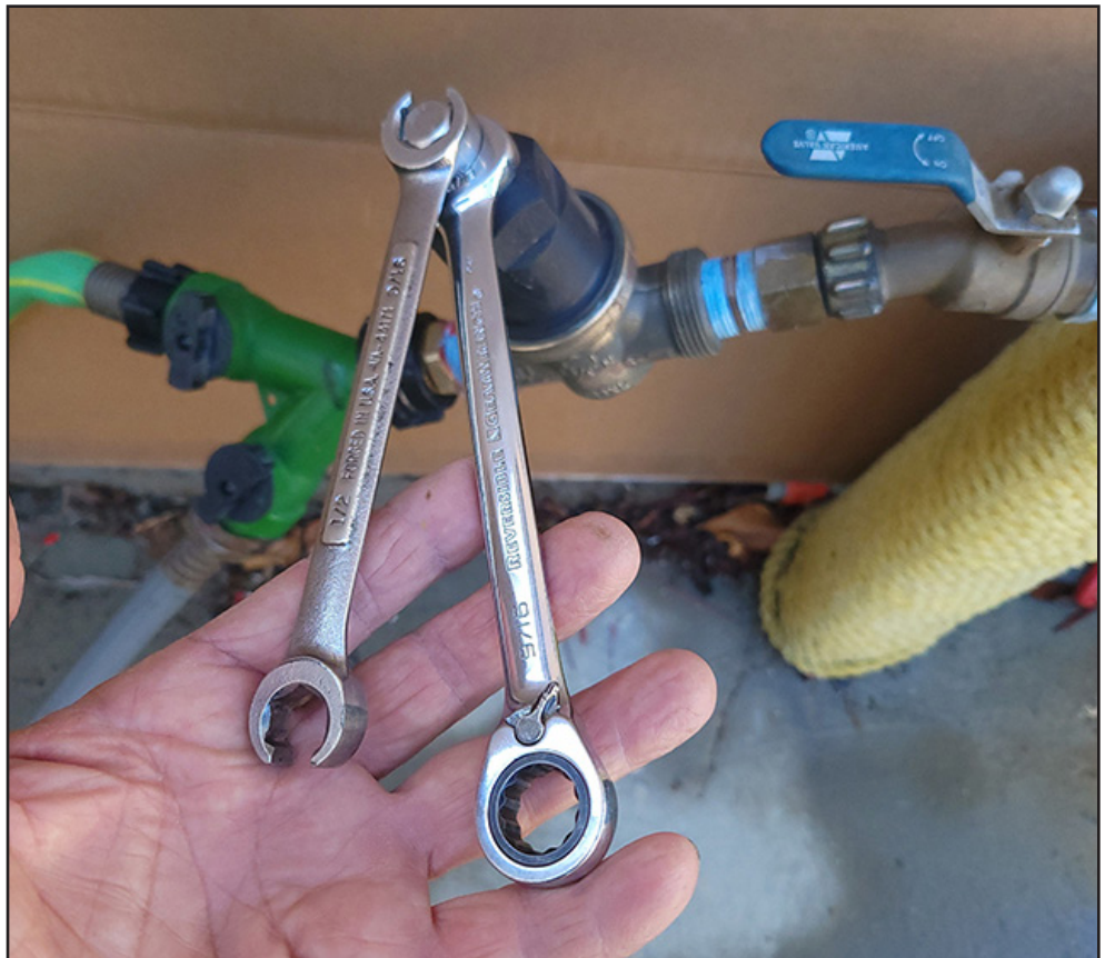
These water-pressure regulators are pre-set to reduce pressure to 50 psi. They can be adjusted for less pressure (you don't want more), if desired, by loosening the set nut and turning the bolt on top of the device while monitoring a gauge.
