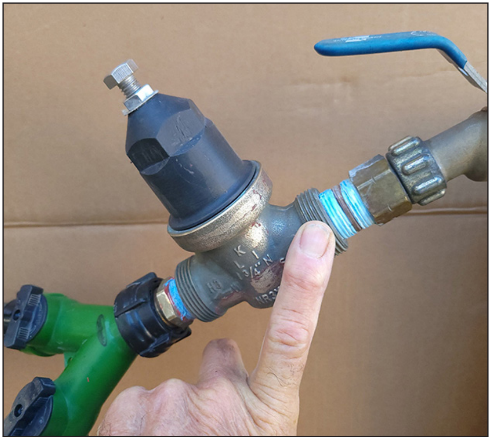
Fittings obtained at a hardware store are threaded into the inlet and outlet, making it possible to hook up to the faucet and a hose that goes to the RV's city water service. Bushings may be required to attach the garden hose thread (GHT) fittings.
