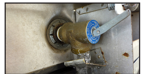
If the pressure-relief valve is leaking, opening and closing the lever a few times might help stop the leak. If not, you'll undoubtedly have to install a new valve. Opening the valve while the water is running out of the drain will improve the flow, aiding in the removal of debris.
