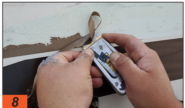
The razorblade scrapers used by V.I.P. Enterprises are more rigid than those often found at hardware stores, giving the technician additional control when removing the vinyl. Made by companies like Stanley, they can be purchased online and at industrial supply stores such as Granger.
