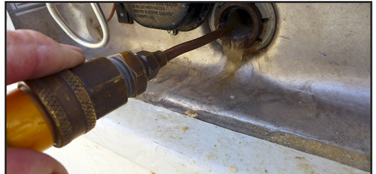
A flush tool will help remove debris and corrosion from the tank. This one is homemade using a few fittings and copper tubing that were laying around the garage. Commercial tools are available online (Amazon) and at most RV parts stores and are very inexpensive. Using push-pull motion (with some added side-to-side action) will dislodge debris inside the tank. Gravity draining the tank alone will not facilitate proper cleaning.
