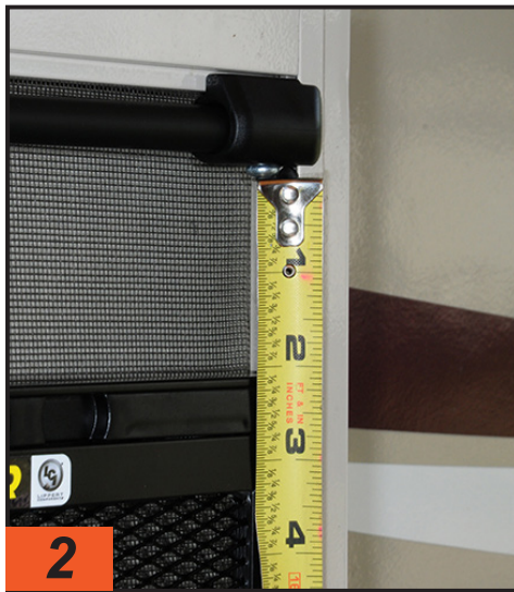
2 In this installation, a 2-inch extrusion was needed, considering the height of the lower section of screen and the location of the previously mounted Screen Shot screen door closer. To make a 2-inch gap filler, two sections of extrusion material were snapped together via the barbed layers of plastic.
