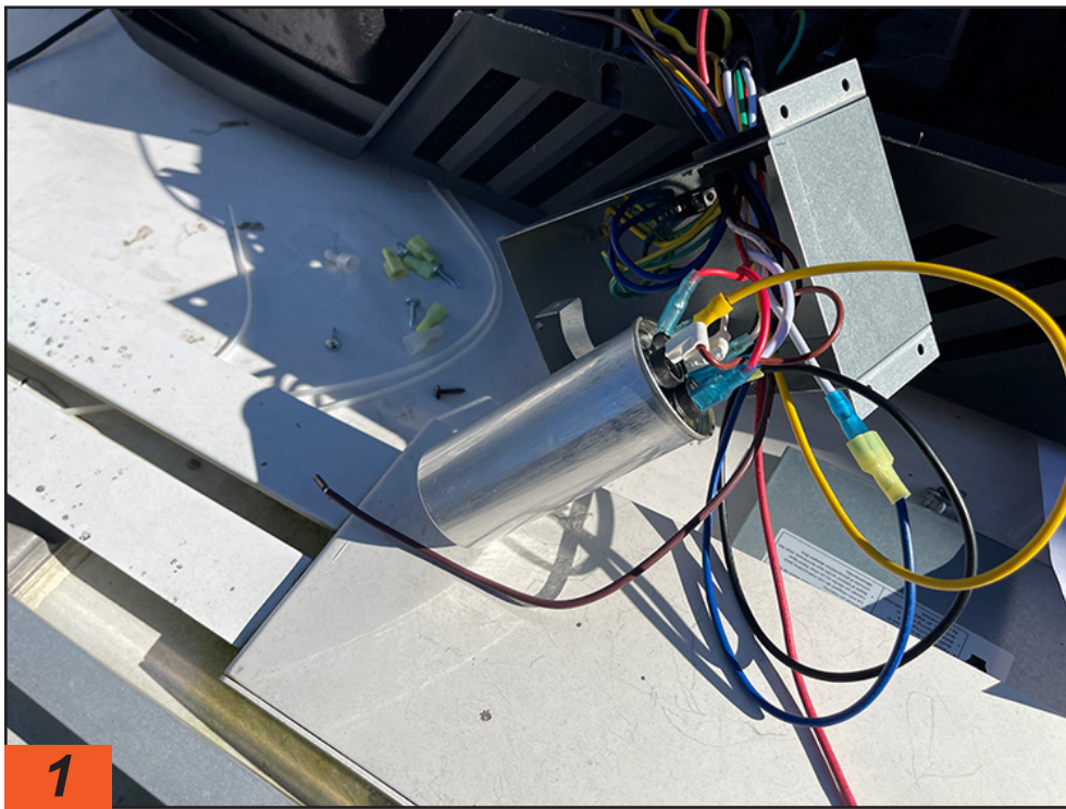
1 Once the cover of the air-conditioner is lifted off, the starter/junction box is removed and/or opened, depending on the brand and model of air-conditioner, and the soft start wires are routed into the box.
