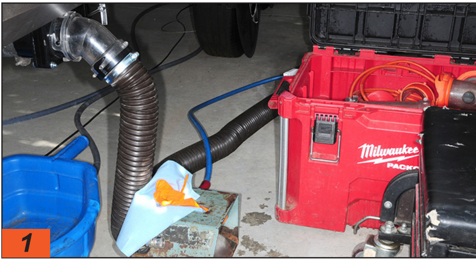
None of the equipment needed to flush the tanks is exotic, but care is taken to make sure no contents are spilled on the ground during the flushing process.
