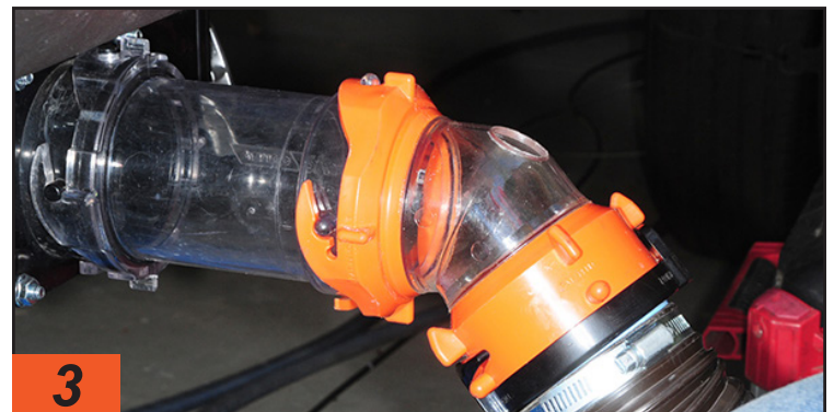
A new elbow fitting configured by RV Flush to accept the hose and nozzle was fit into place. The clear plastic elbow provides the best possible view of the process. This type of observation is not for everyone.
