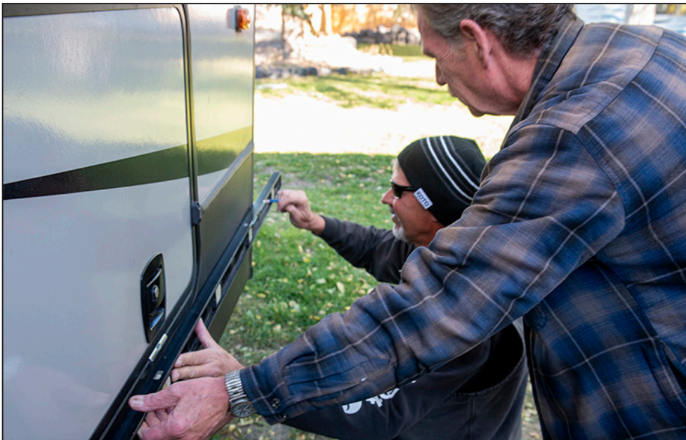
Kevin Jorgensen (kneeling) has been making and installing RV skirting in southwestern Idaho for 20 years. Larry Jones helped install the skirting on my 39-foot Sprinter fifth wheel. It was a three-day job, with a third of that spent taking precise measurements.
