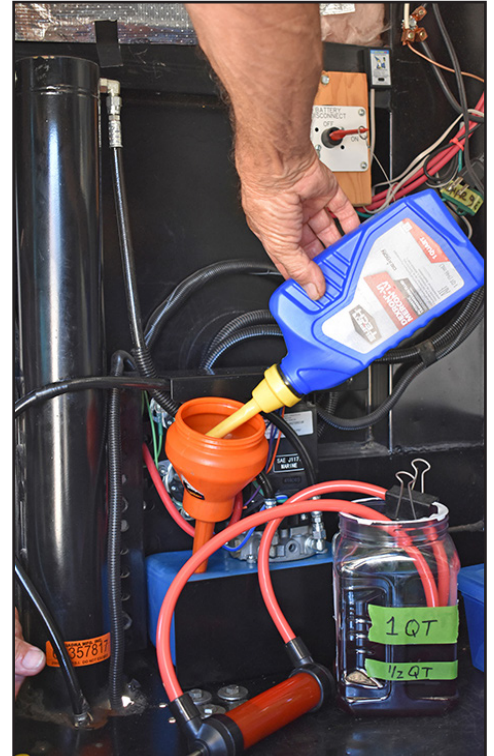
Top off the reservoir with the automatic transmission fluid specified by the system manufacturer before wrapping up the project. The additive may not work perfectly, but it will likely mitigate most of the unnerving popping noises. Noises were eliminated on this fifth wheel. RVE
