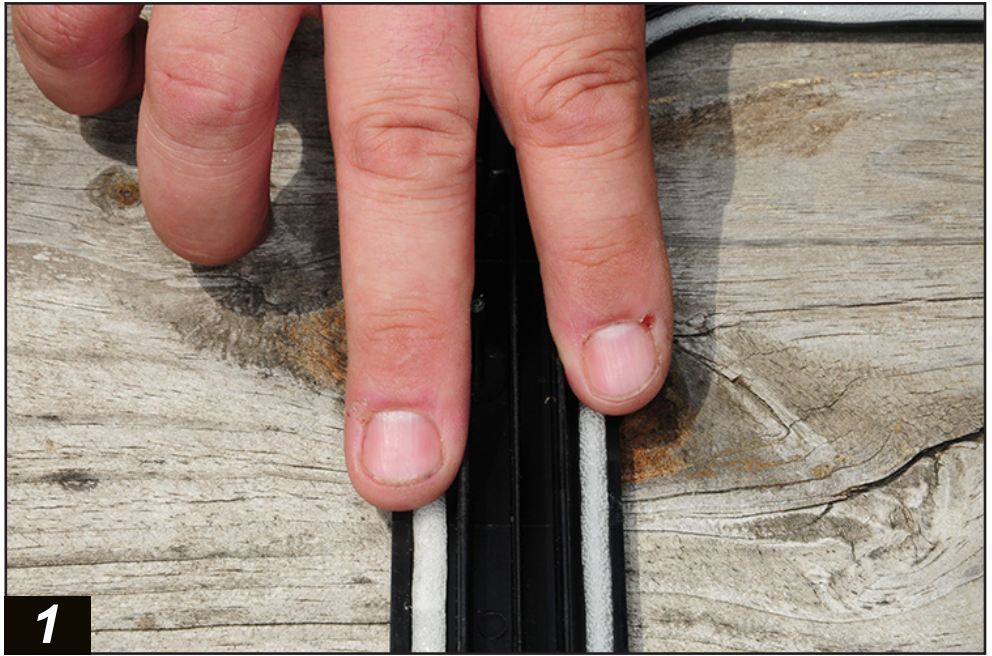
We decided to tackle the window replacement first. To make things easier, strips of sealer to seat the window glass are pre-installed in the outer frame.
