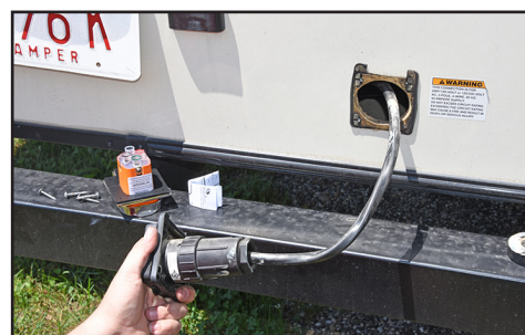
The receptacle replacement process is pretty straightforward. If you have enough cable, you can just cut the old receptacle off and strip the new wires accordingly. You can also disassemble the old one and — provided it isn't internally broken like the one in this test installation — you can save the step of stripping the cable.
