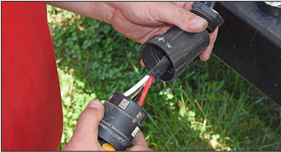
Once disassembled, a broken screw for the L1 hot leg was identified. There was also a stray wire sticking out of the neutral terminal.
