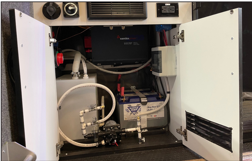
The finished project gives a glimpse into the complexity of the system. The entire water system was removed and re-engineered for the space. The Battle Born LiFePO4 batteries were secured to the floor with a custom mounting system and strap. The rest of the components were mounted above and behind the batteries. The original battery switch was too small to handle the loads, so a new, larger switch was installed. The original converter was removed, turning the bottom of the fuse and breaker panel into an air vent. An additional air vent was cut into the cabinet door.
