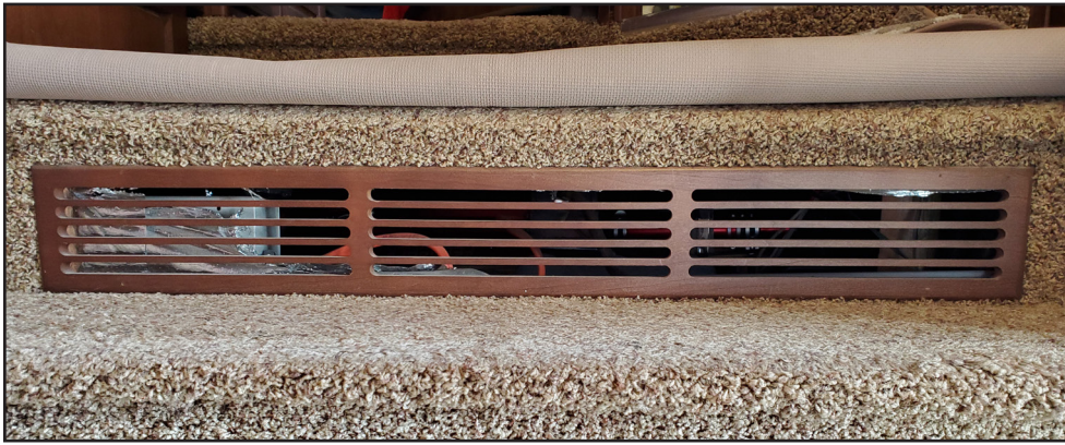
Return air vents can be found in various areas in RVs. This vent is cut into the steps that lead to the bedroom in a fifth-wheel. It's important to keep the area around the return air vent free of stored items. Any obstruction can diminish the efficiency of the furnace.
