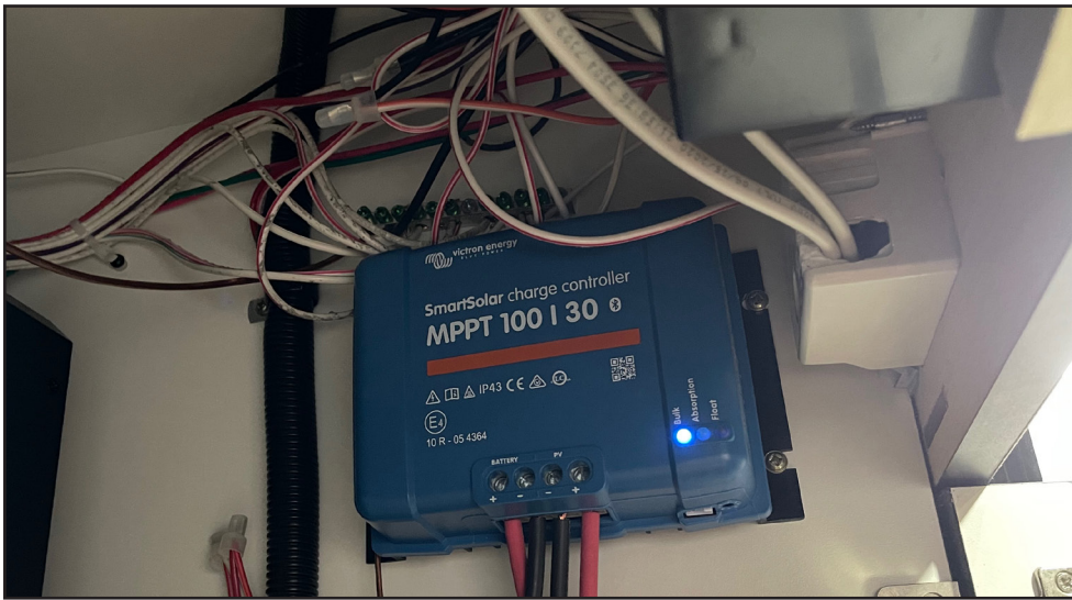
Once completed, the Victron SmartSolar charge controller is tucked up out of the way and fully functional.
