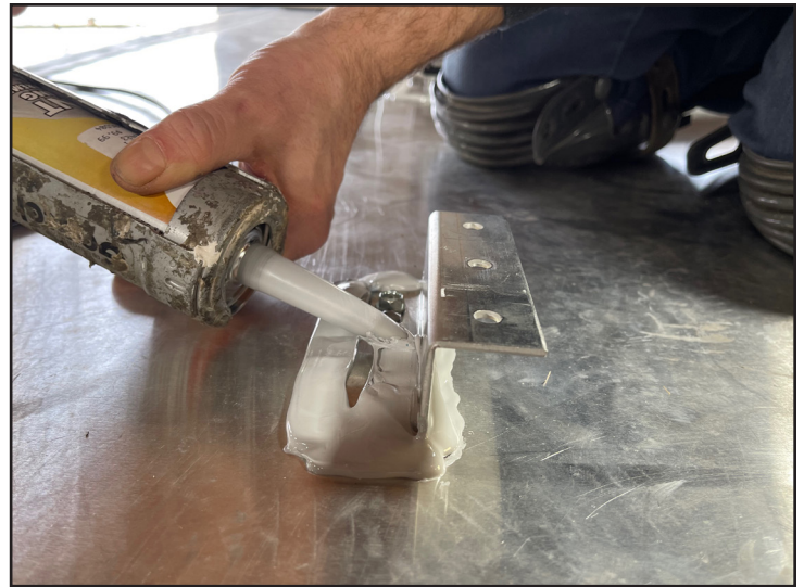
Be sure to use plenty of sealer that’s appropriate for the particular type of roof. Do it right the first time, because the panels are a chore to remove and reinstall, as is resealing the brackets.
