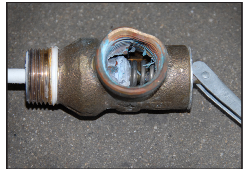
Here is a good example of a frozen emergency relief valve. Note the calcium deposits and rust that eventually prevented the valve from functioning.
