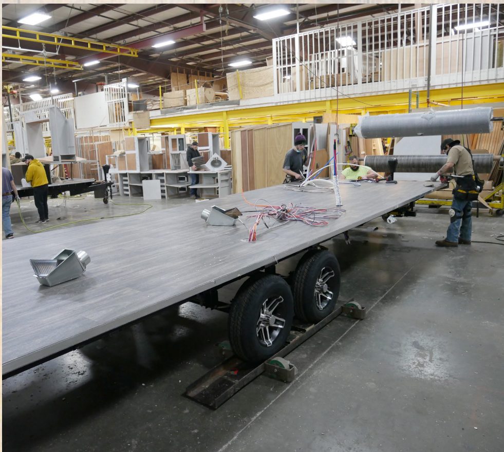
Keystone technicians prepare a floor to receive the rest of the house build after laying down laminate flooring atop the Hyperdeck.
