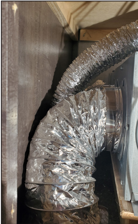
Inspect all ducting from the furnace for integrity. Cuts or cracks will reduce efficiency because the heat will escape before reaching the registers. Furnace manufacturers require a specific number of flexible ducting runs and/or the use of a plenum. It may be possible to repair small areas with certified metal duct tape, but in most cases the tubing will need to be replaced.
