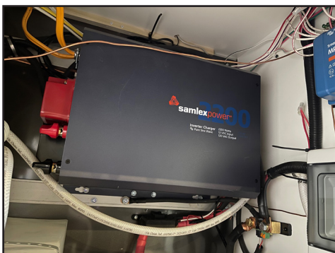
The inverter/charger is a sizable unit, which required building a mounting frame from the wall stout enough to secure the unit.
