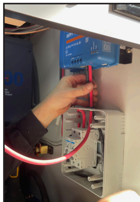
The equipment was tough to mount in such a tight space and required Turner to become a ninja to get in there and do all the work.
