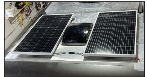
Topside, the clean installation will provide 320 watts of solar power. Along with the 30-amp MPPT charge controller, 2.2kW inverter system and 210-amp-hour lithium battery bank, the panels will deliver more than enough power for the trailer's intended part-time use as a mobile workshop and sometime guest quarters.
