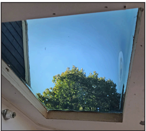
Moving to the inside, we had a couple of options. First was to custom order a thin inner dome from Icon Direct that would match the depth of the roof and dome. Icon makes them in 2-inch and 5-inch depths, as well as custom models. For our installation, however, we opted to eliminate the inner dome.
