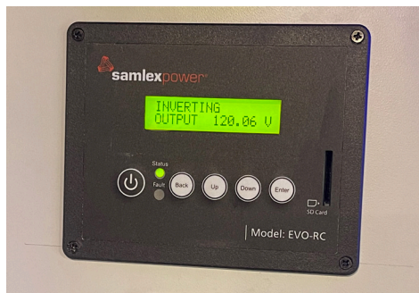
The Victron battery monitor is also viewable and controllable via a remote panel, which was installed along with the Samlex inverter/charger remote panel in the galley.
