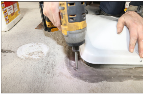
The sealant topside is dirty and the skylight is badly weathered and broken, the victim of an earlier cob job. As seen on this roof vent, removing the sealant from the skylight itself isn’t necessary when replacing the skylight as long as you can expose and access the screws for removal.
