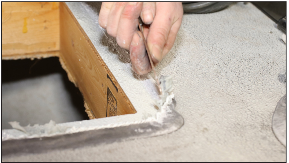
Once the skylight is off, remove as much of the remaining sealant as you can without damaging the roof. Warming the sealant can help.
