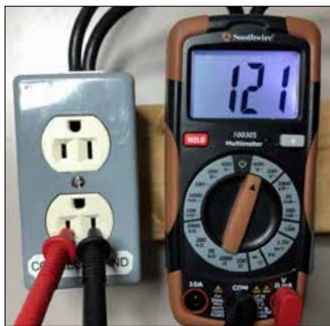
As seen in this photo of an outlet being tested in the author's test lab, a multimeter can be used to check voltage in your RV as well as checking the proper voltage in a park's electric pedestal.
