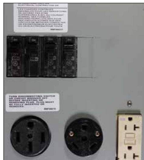
A typical campground electric pedestal with 50-, 30- and 20-amp connections.
